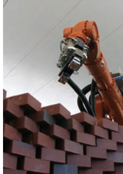
II_ Programmed robot building up the brick wall © Gramazio & Kohler, ETH Zürich
